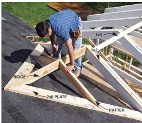
The new roof extends onto an existing roof using a ridge board. No loads from the new roof are transferred to the existing dwelling. The existing roofing has not yet been trimmed.
